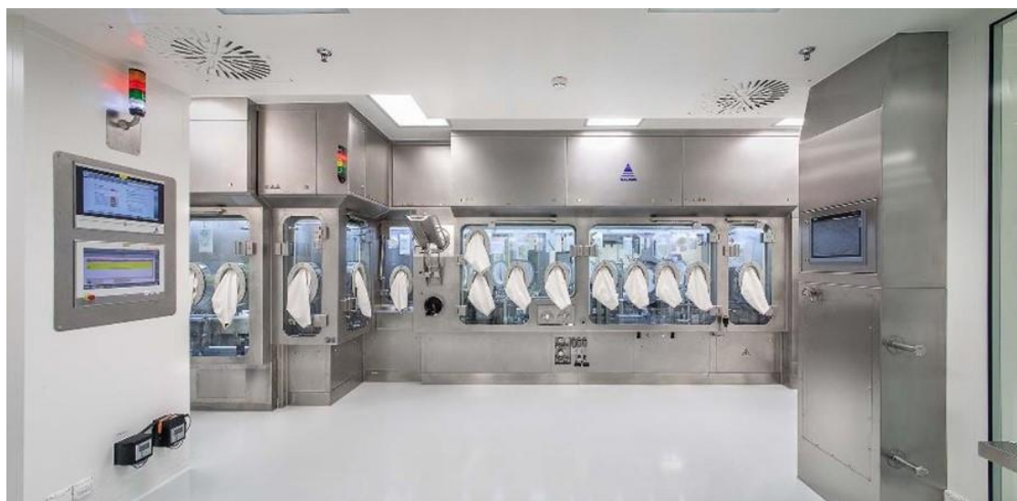
Figure 1 Isolator with glove interventions
